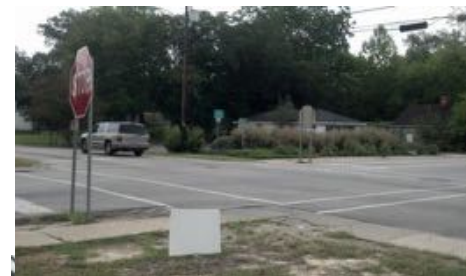
Sidewalk Maintenance Issue
