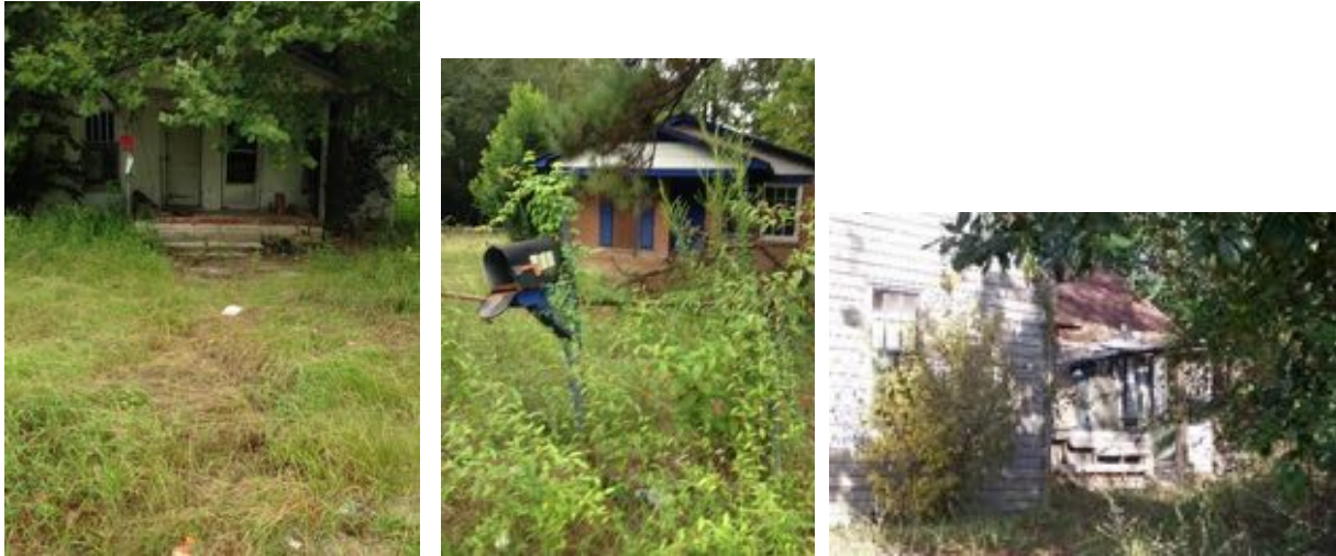
Figure 13: Deteriorated or dilapidated homes in South Hartsville
